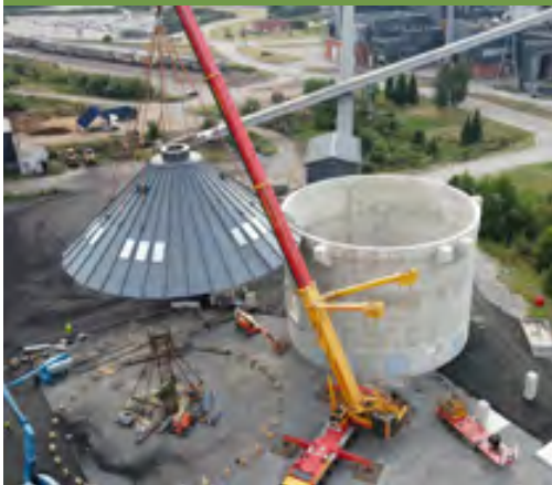
Installing the cap on the silo that now stores biofuel at Kirkniemi Mill, a major achievement on Sappi's decarbonisation journey
